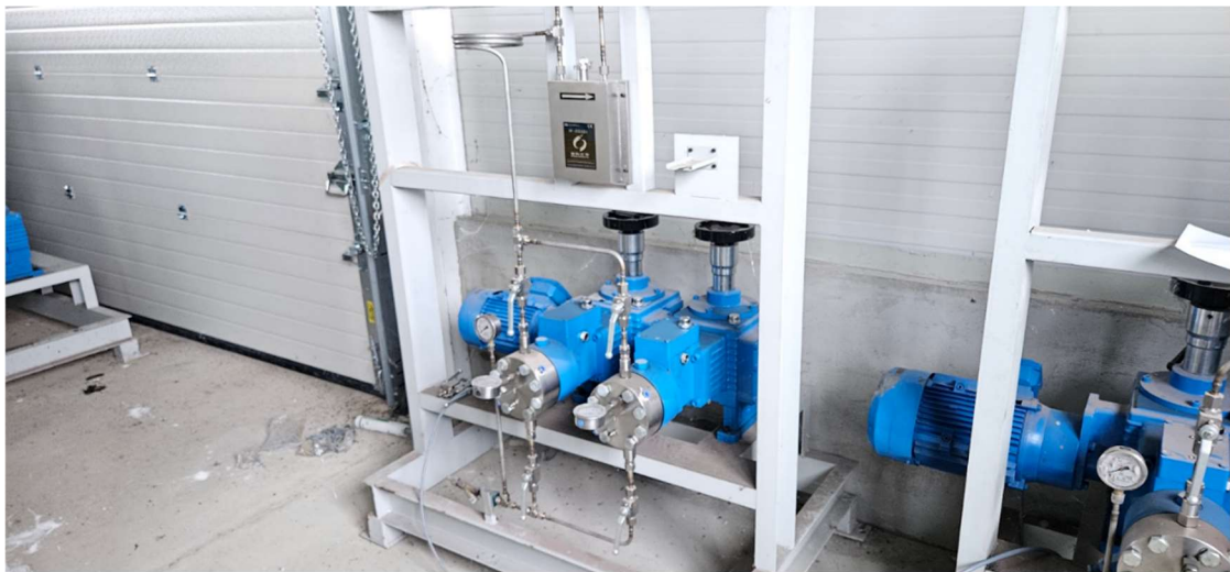
7. Dosing unit for ethanol
